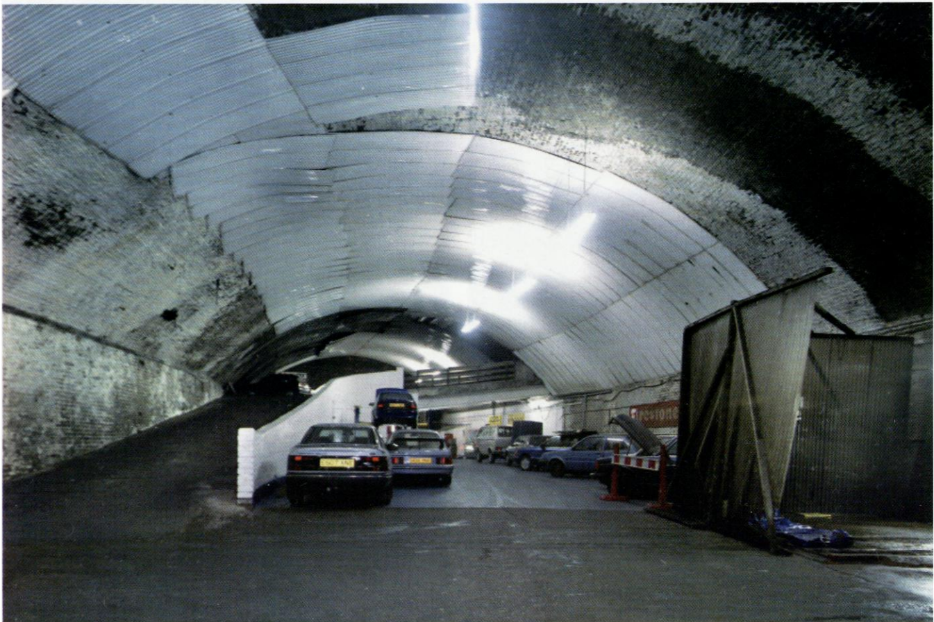
The site of the former Dingle Station on the Liverpool Overhead Railway. The station tunnel has been converted into a car repair workshop. A roof collapse occurred here in July 2012. Photo Nick Catford
